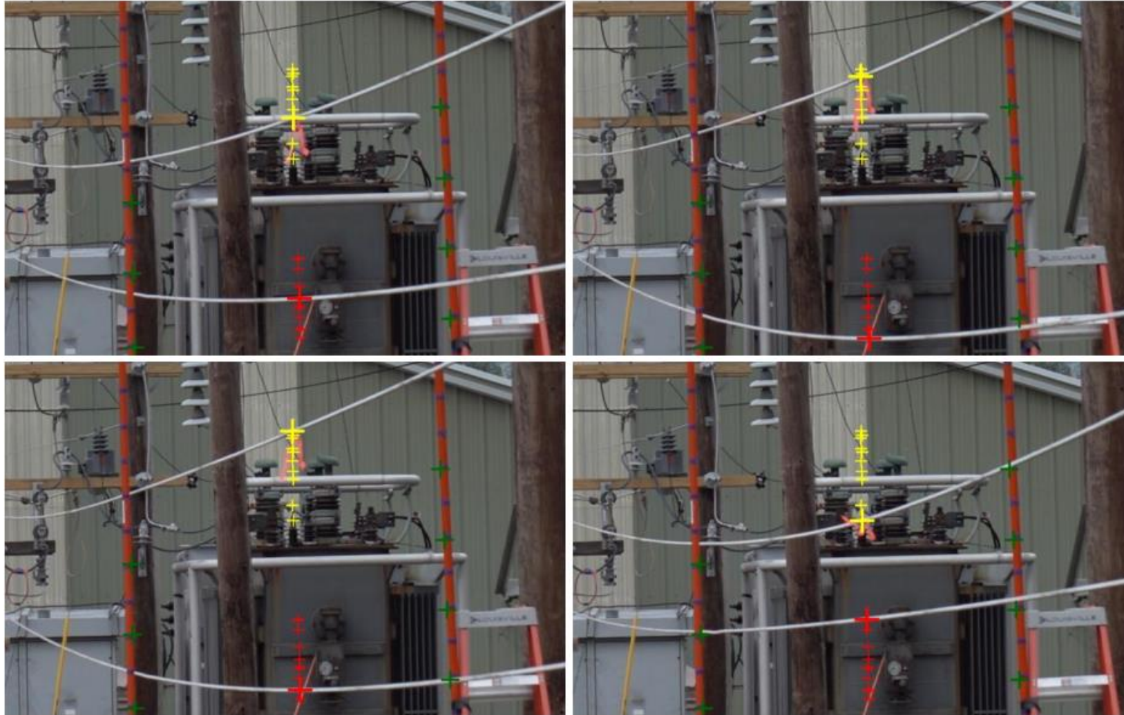
Event 10290: I = 2955 \text{ A} ; t = 27 \text{ cycles} ; vertical separation = 30 in span = 200 ft; sags = 24 in; 336 ACSR
